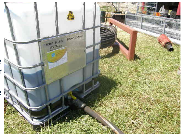
BluBac dosing the bore via cam lock connection
